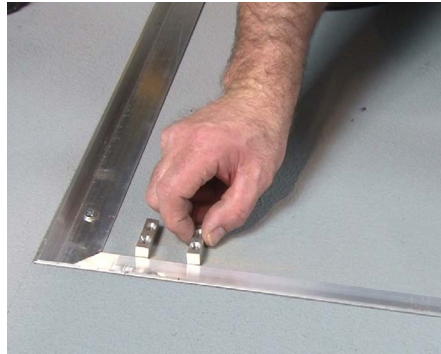
17 Roll back the mat. Using the recorded dimensions, mark the locations on the concrete, off-set from the frame.
