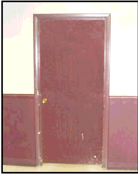
Damage to unprotected door and frame
